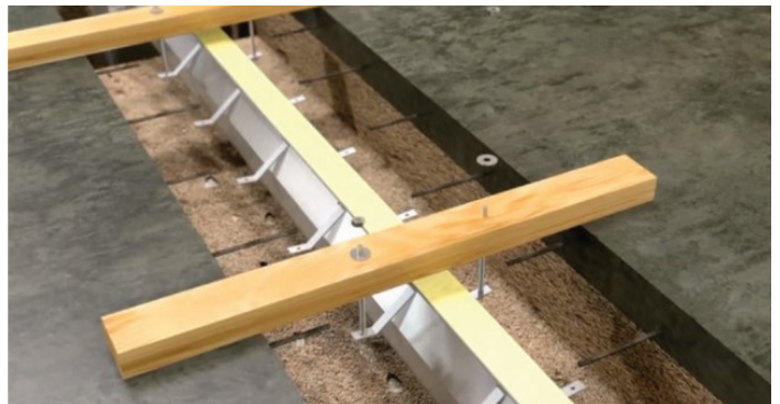
WOODEN PIECE PLACED ON THE DRAIN
