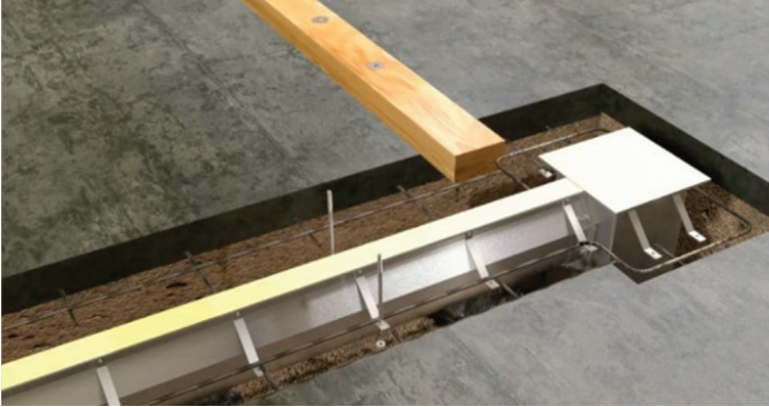
WOODEN PIECE REMOVED FROM THE DRAIN
